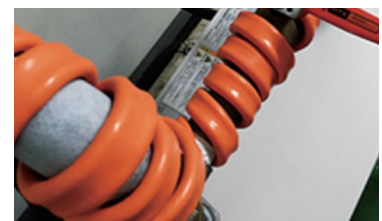
Heat Retention on Pipes (flexible along pipes)
